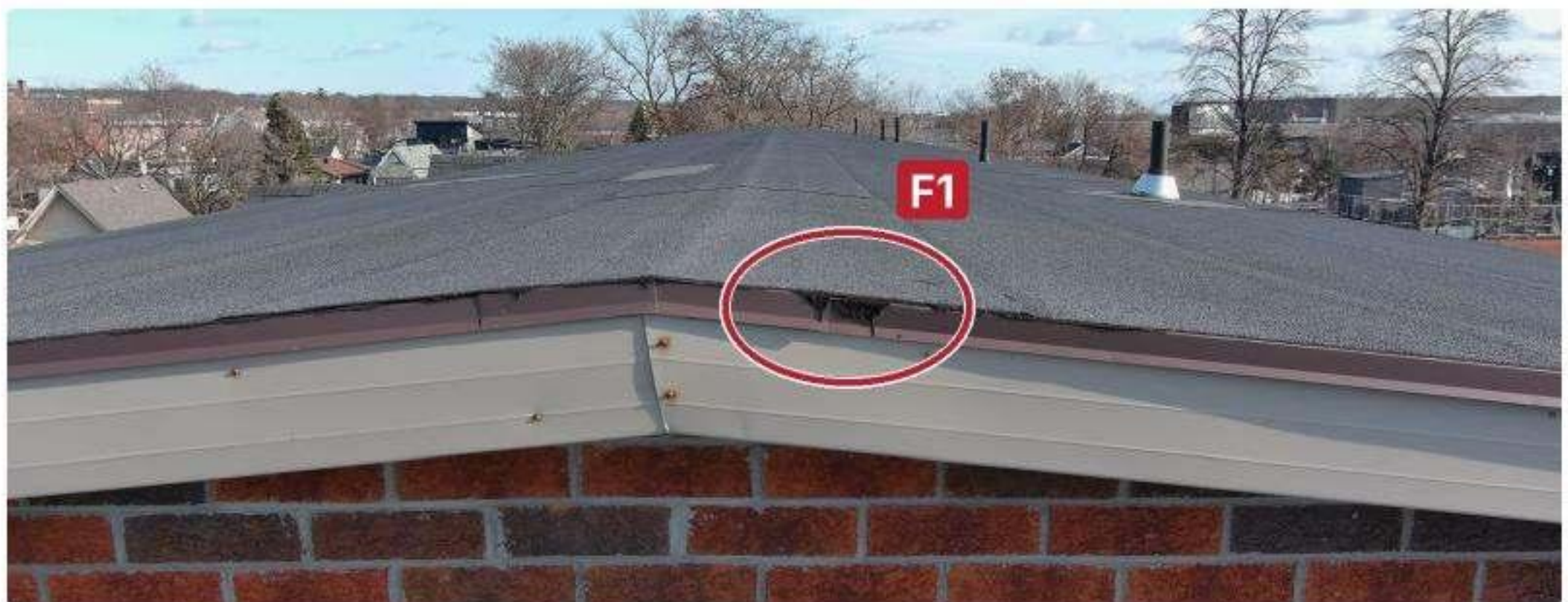
F1.1 – Lifted, open membrane edge at the corner of the end wall.
