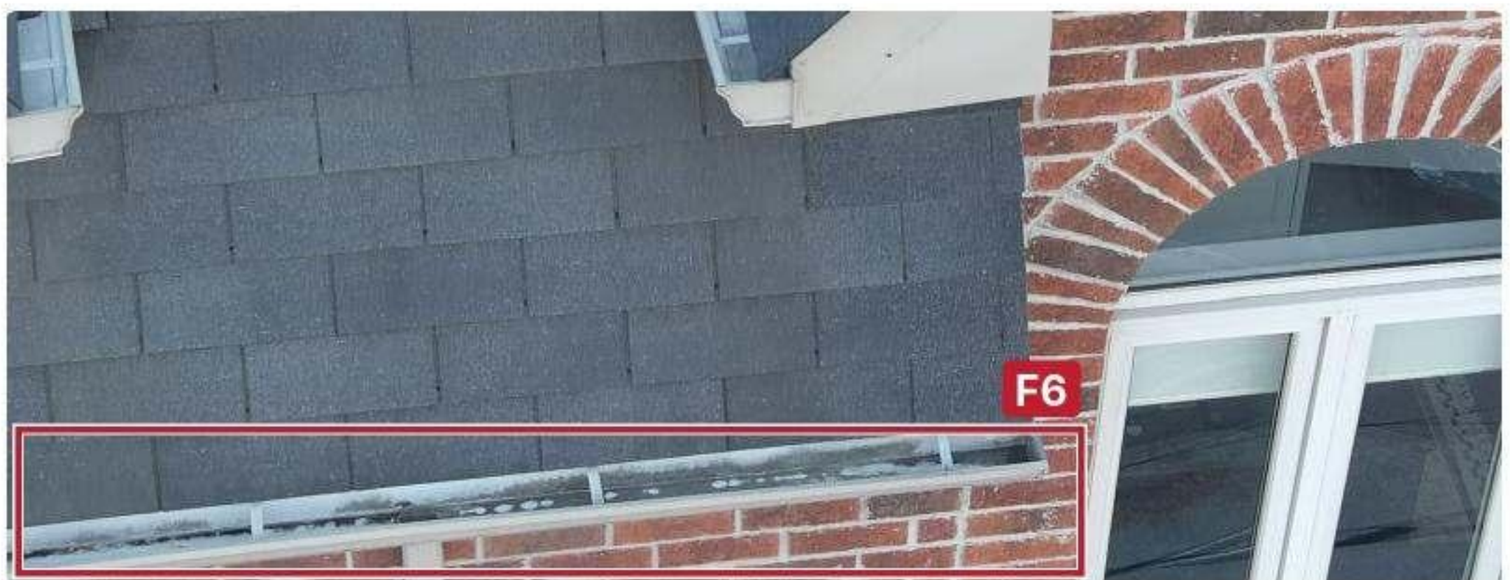
F6.2 – Debris in a dormer-level gutter.
