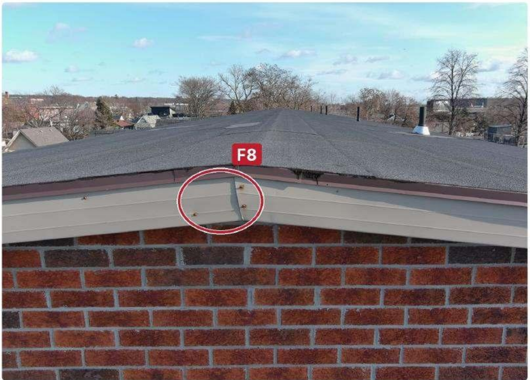
F8.1 – Rust-stained screw heads on the gable-end trim.
