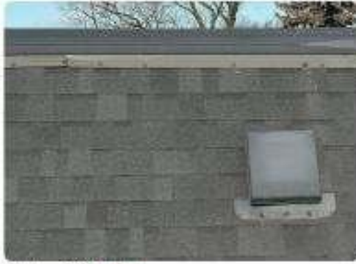
Photo 120 · F4 Rear slope close-ups
