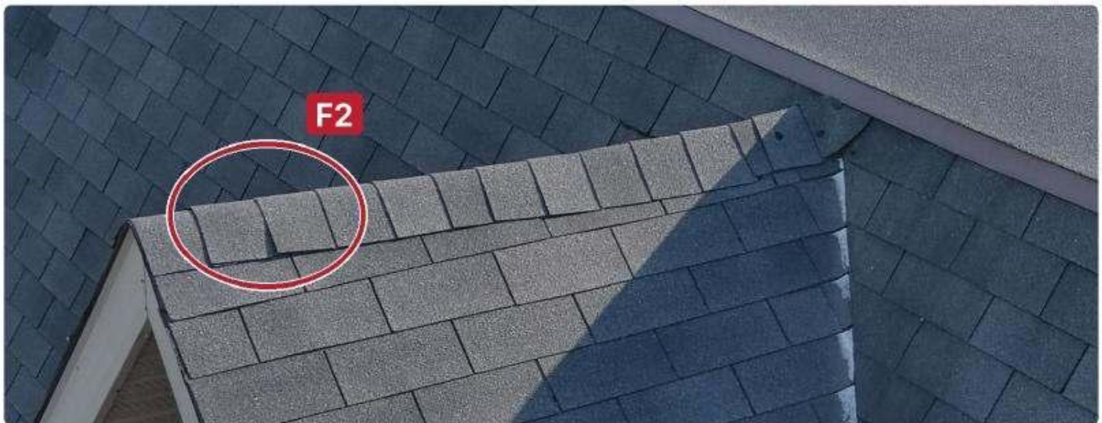
F2.1 – Raised ridge-cap shingle at the dormer ridge.
