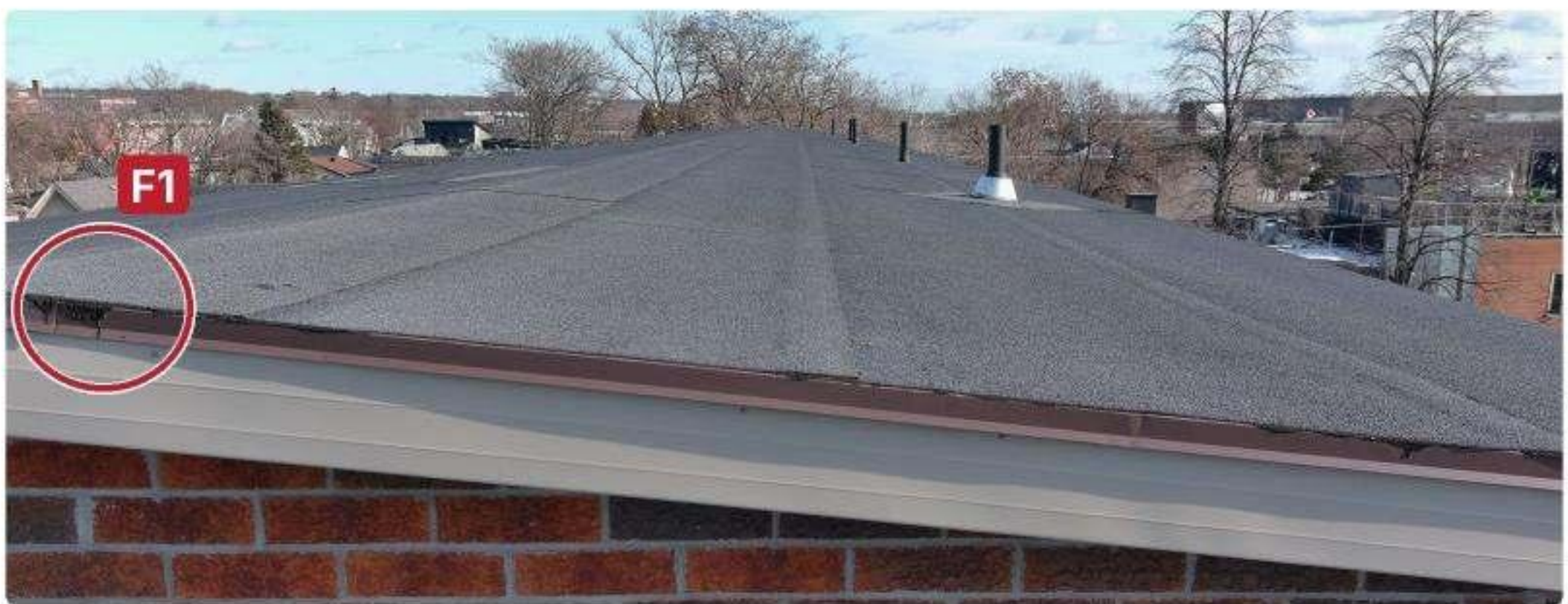
F1.2 – Irregular edge with exposed bitumen along the perimeter flashing.
