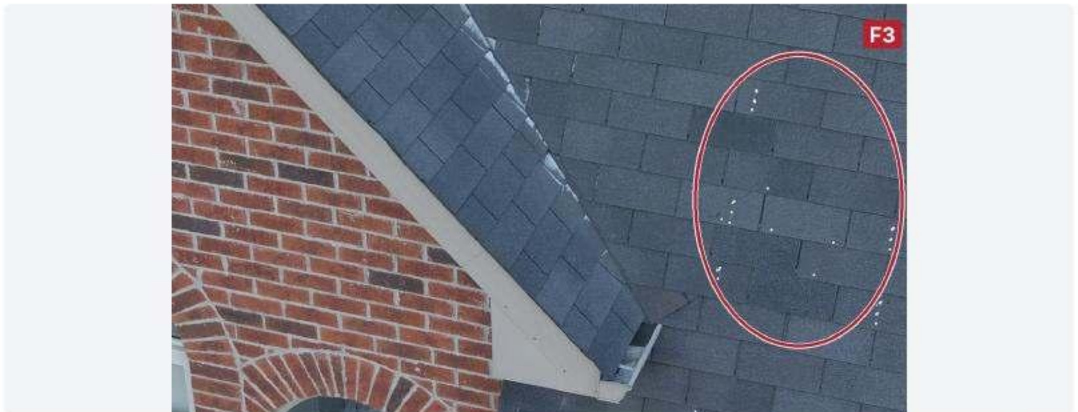
F3.1 – Rows of exposed fasteners / sealant dabs and a mismatched replacement shingle.
