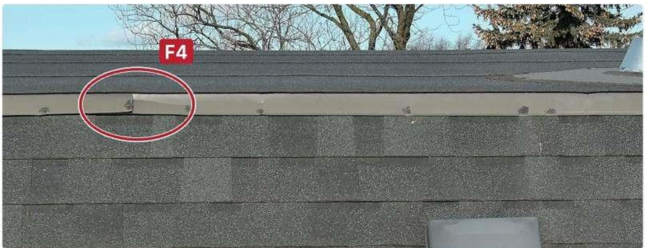
F4.2 – Raised / buckled flashing lap joint.
