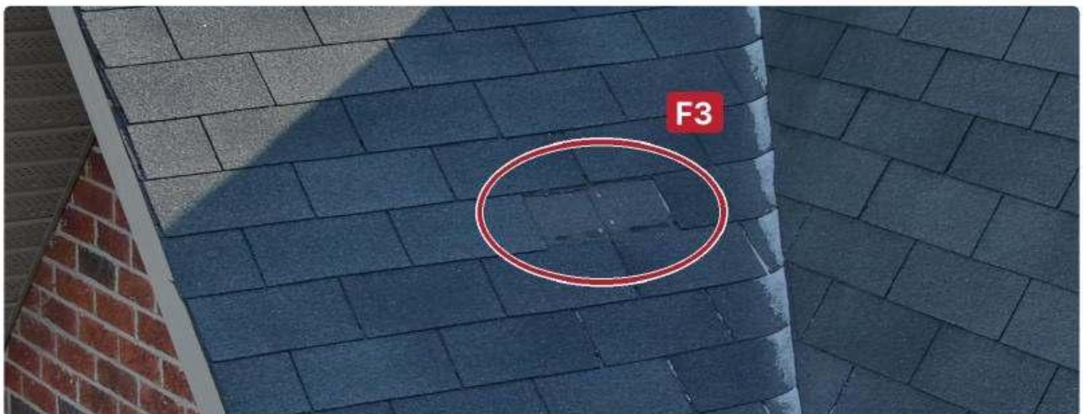
F3.2 – Repaired shingles with face nails and a visible tar line.
