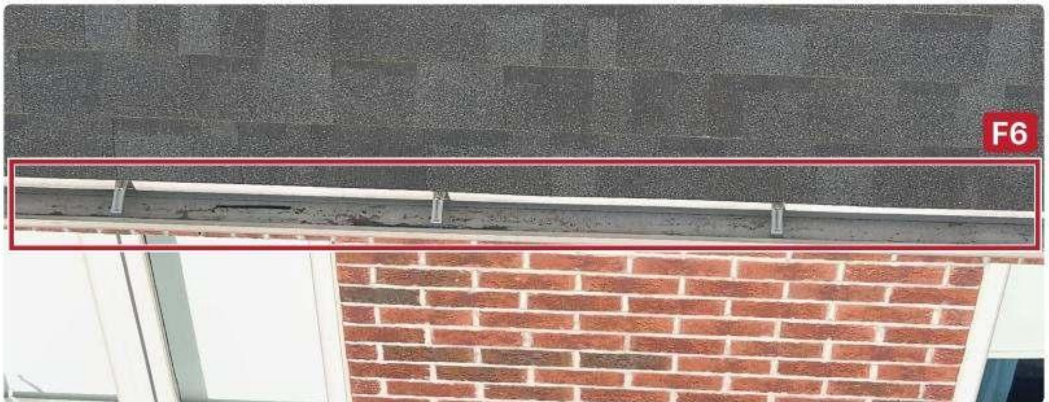
F6.1 – Sediment and debris in the rear eavestrough.
