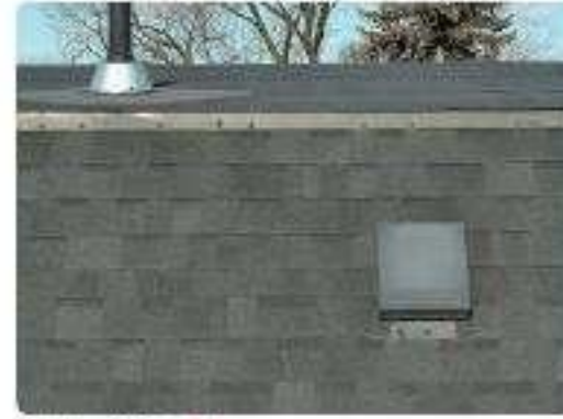
Photo 122 · F7 Rear slope close-ups
