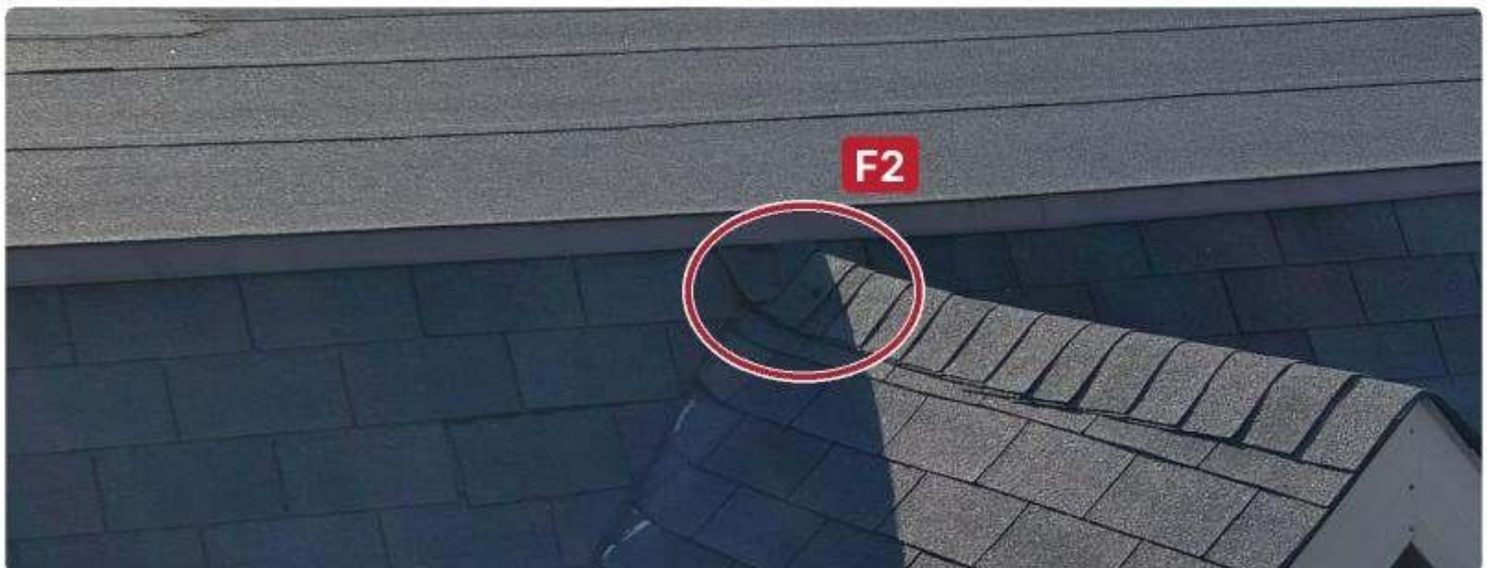
F2.2 – Raised cap shingles where the dormer ridge ties into the main slope.
